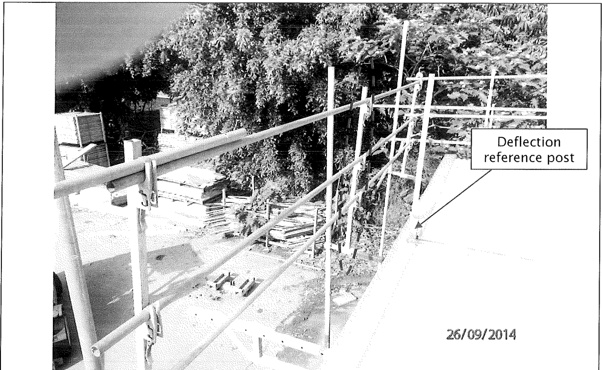
Figure 3 Deflection reference for Metal Fascia Bracket System Tests 3-Rail EP posts and rails. The reference for deflection is a removable post (arrowed) secured to the roof structure. The middle post to be tested is 'circled'.
