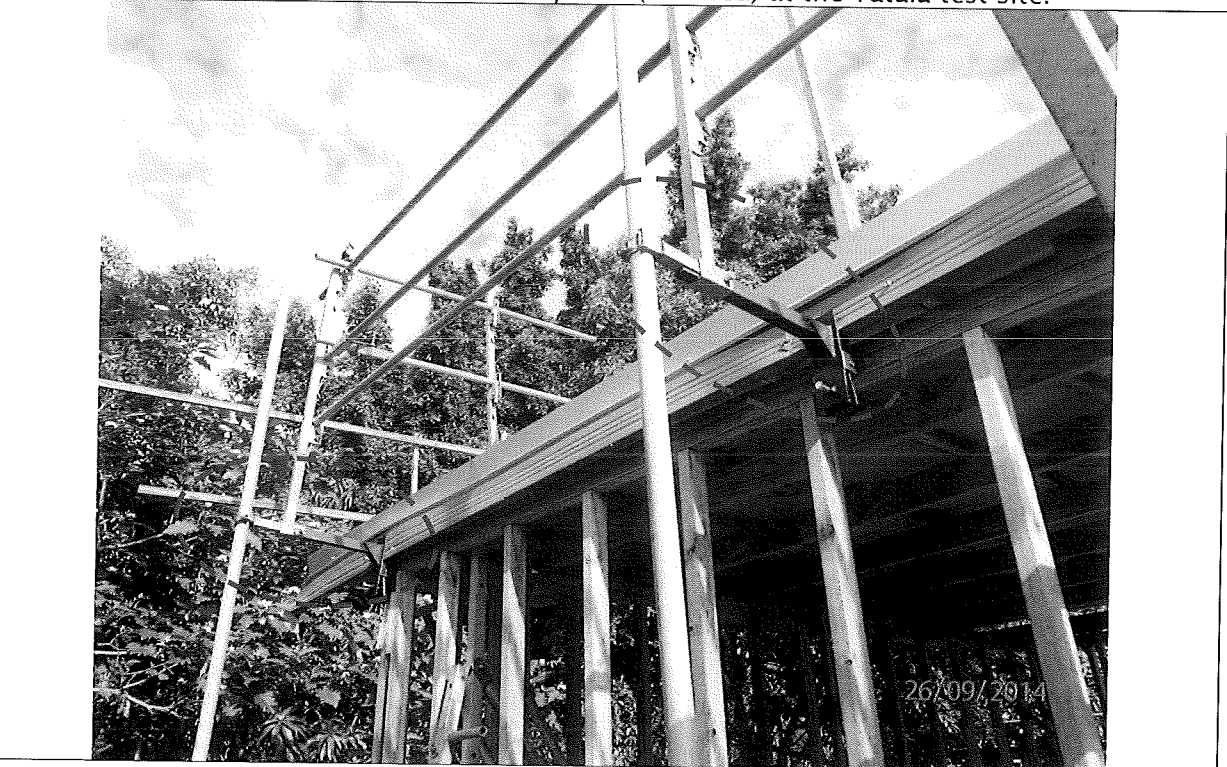
Figure 2 Metal Fascia Connection to Pole Detail of the Metal Fascia Bracket attachment to the fascia and pole.
