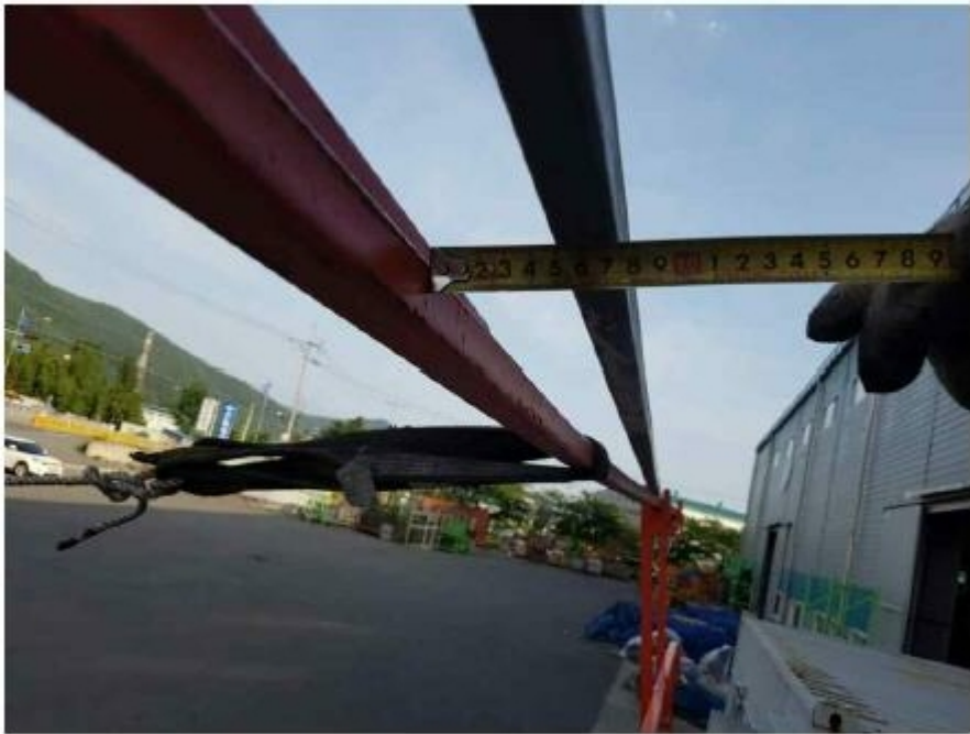
Figure 11 -50mm deflection measured at center of Top Rail Span
